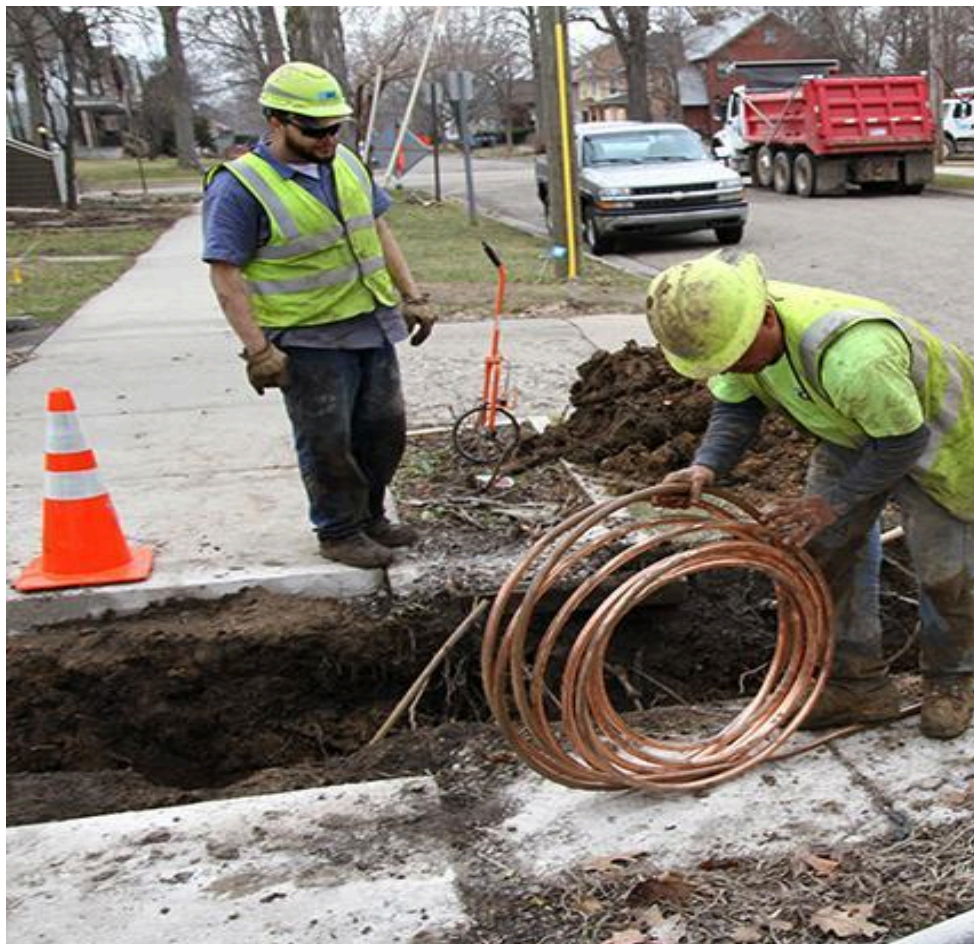
Figure 3: Close-up on the process of the water supply's replacement plan, swapping the lead pipes with a more sustainable and safer material, copper.
